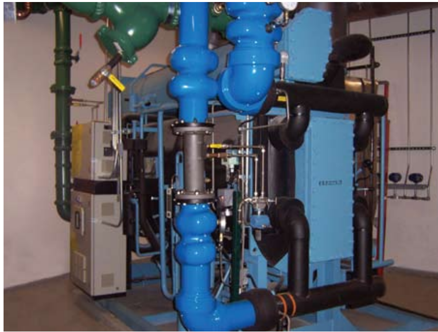
Thermax® absorption chillers.
