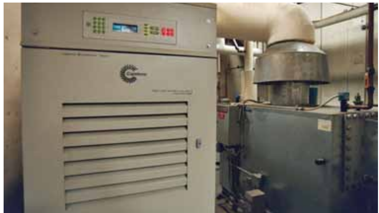
A Capstone microturbine provides electricity, cooling, and heating to Citibank in La Jolla.
