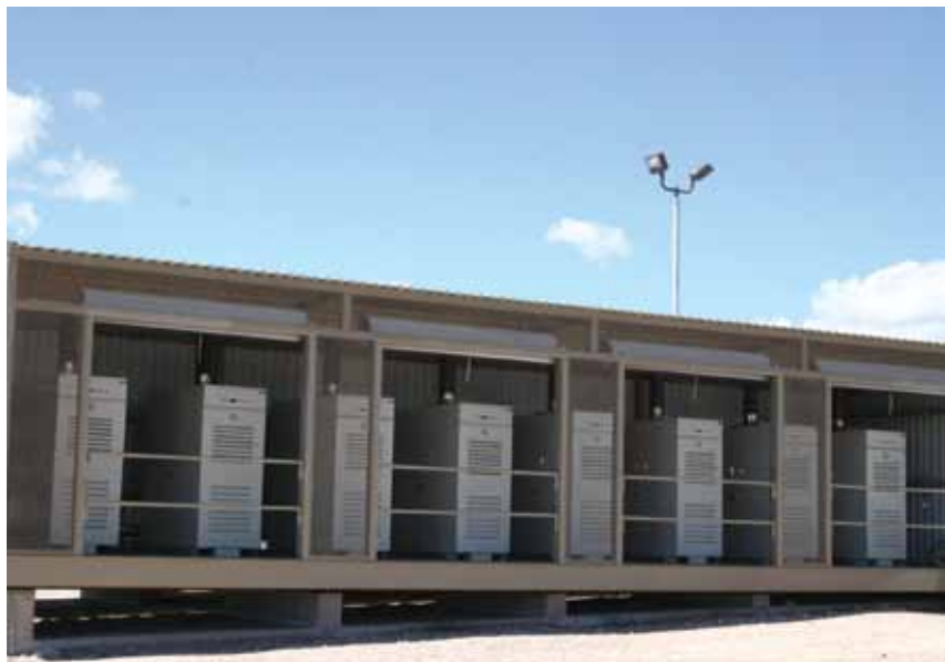
Fifteen 65kW microturbines provide the primary power for this oil pipeline booster station in New Mexico.
